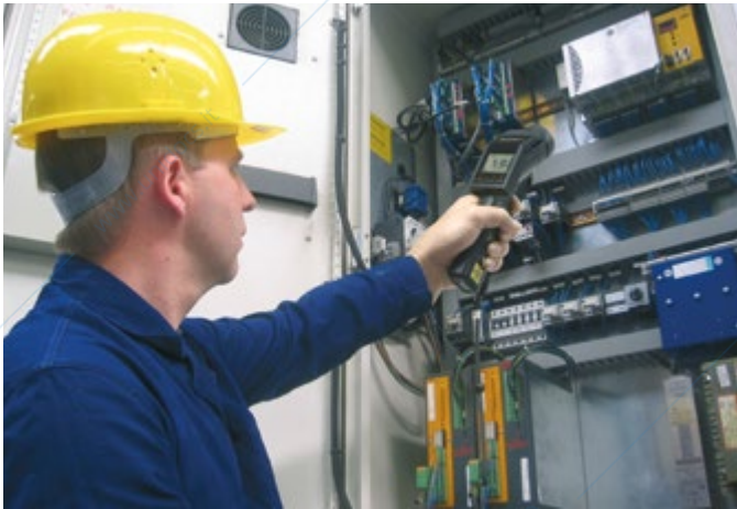
Detailed infrared temperature measurement of an electric control with the help of the installed close focus optics for 1 mm ranges of the optris® LS
